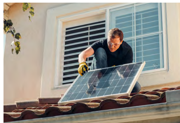
Rooftop solar. Source: Kindel Media, Pexels.
